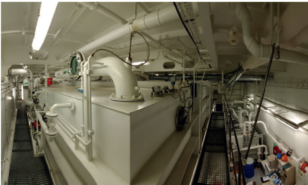
EXISTING ADVANCED WATER TREATMENT SYSTEMS CAN BE CONVENIENTLY UPGRADED TO THE NEW CS-MBR STANDARD
